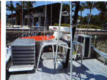
Rooftop power and air con
