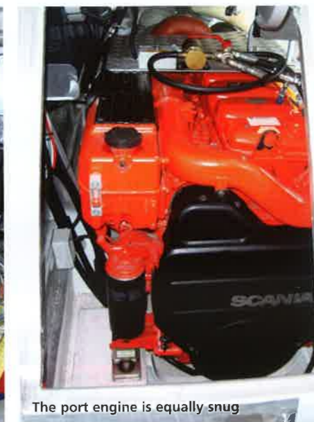
The gen-set is tucked up aft in the engine room
