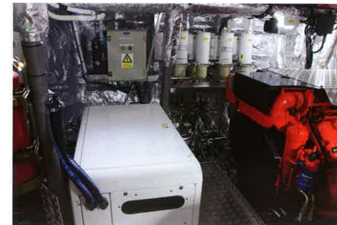
Engine room and gen-set
